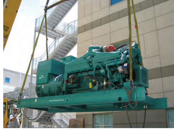
Cranes were used to lift pieces of the generator sets into the installation space.
