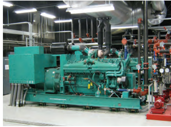
Cummins installed one DQGAB 1500 kW and two DQGAA 1250 kW generator sets.
