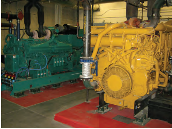
One challenge was paralleling a Cummins and Caterpillar generator set.
