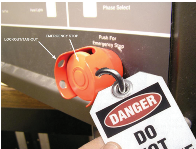
An emergency stop switch fitted with lockout/tag-out provisions.
