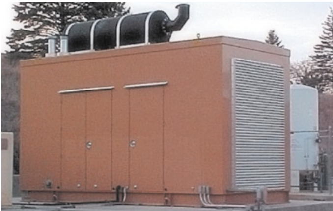
This skin-tight generator enclosure at a hospital in Audubon, Iowa, features access panels for ease of maintenance and a residential exhaust silencer for minimizing generator noise.
