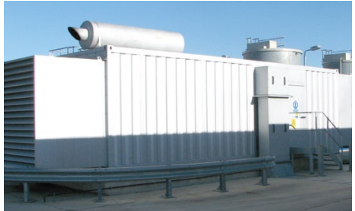
A walk-in enclosure at a regional hospital in Swindon, England, houses a new generator installed when the hospital expanded.
