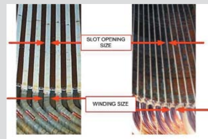
Figure 1 - Winding and slot size comparison shows that for similar winding size, the slot size of a wire-wound machine will be much smaller, resulting in lower harmonic distortion in voltage produced.
